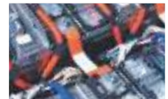
Connection resistance of battery busbars
